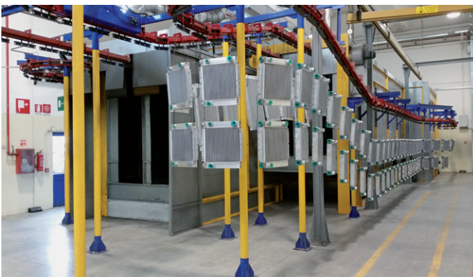
Paint shop (powder coating)
