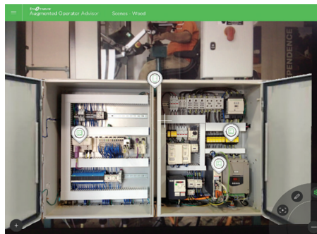
Virtually-open electrical cabinet
