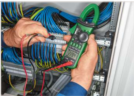
Current measurement in the switchgear cabinet
